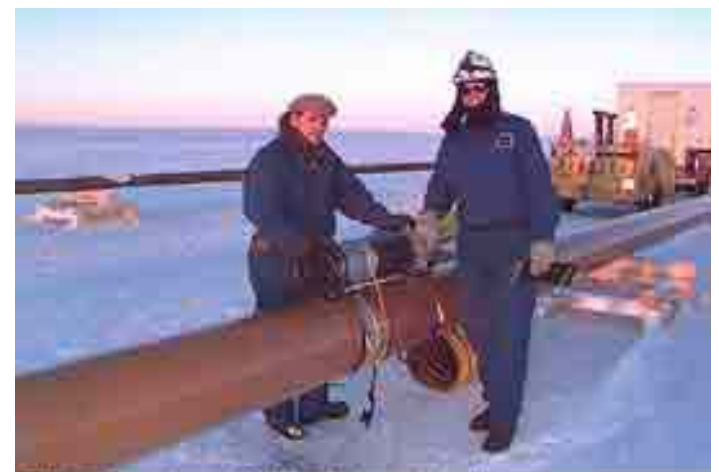
Photo Courtesy of Yxlon International
